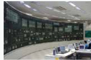
Remote supervisory controller for electric power system control station
