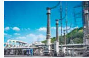
550kV gas insulated switchgear
